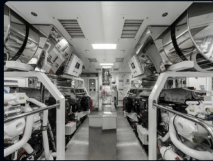
Protect the Vessel Machinery
